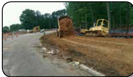
Placing fill dirt that was cut from Bioretention pond to build shoulders and slopes on Sandy Forks Road
