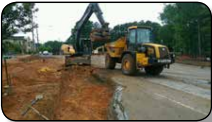
Sunrock crews cutting out a section of Sandy Forks Road to be widened
